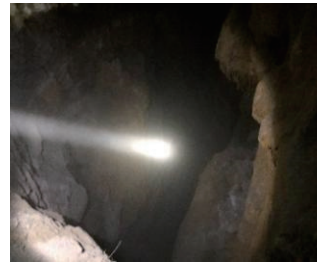
图 1 隧道仰拱下伏溶腔 Fig. 1 Underground cavity of tunnel invert
